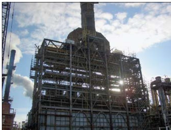
FIG. 4 The convection box after demolition; the skeleton is available for new construction to begin.
