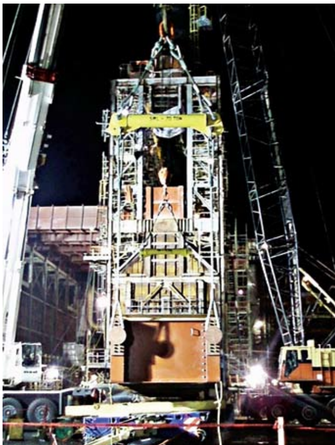
FIG. 6 Module 1 is erected and Module 2 is being lifted. Both cranes use trolleys in the background.
