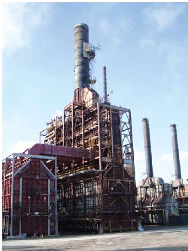
FIG. 1 The radiant sections and convection section of the Come by Chance refinery were deteriorating due to severe North Atlantic climate.
